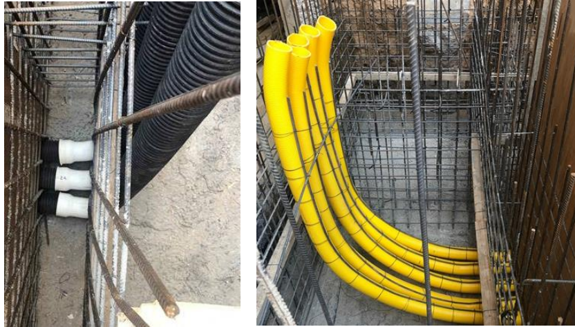
FIG. 14. General services piping
