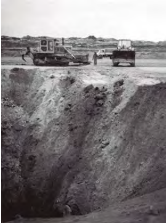
Crater left by a 1,000 lb. bomb dropped by the Vulcan on 1 May. The heavy machinery of the Construc- tion Squadron is shown filling the big hole in the ground
